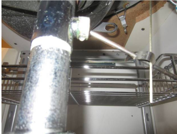
Drip leak noted at stopper mechanism under sink.
