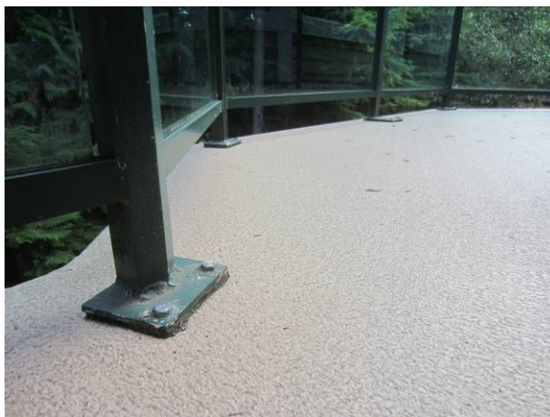
Recommend sealing around balcony railing penetrations.
