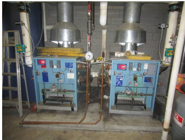
Hot water boilers.
