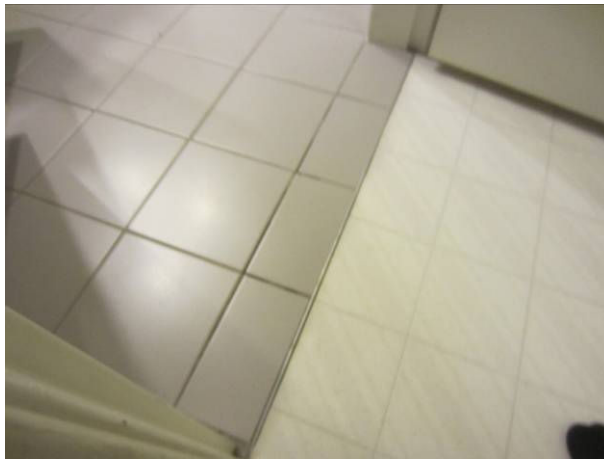
Cracked grout noted to bathroom floor tiles.
